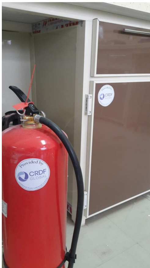
Fire extinguishers before and after installation
