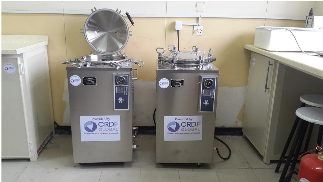
Autoclaves before and after installation
